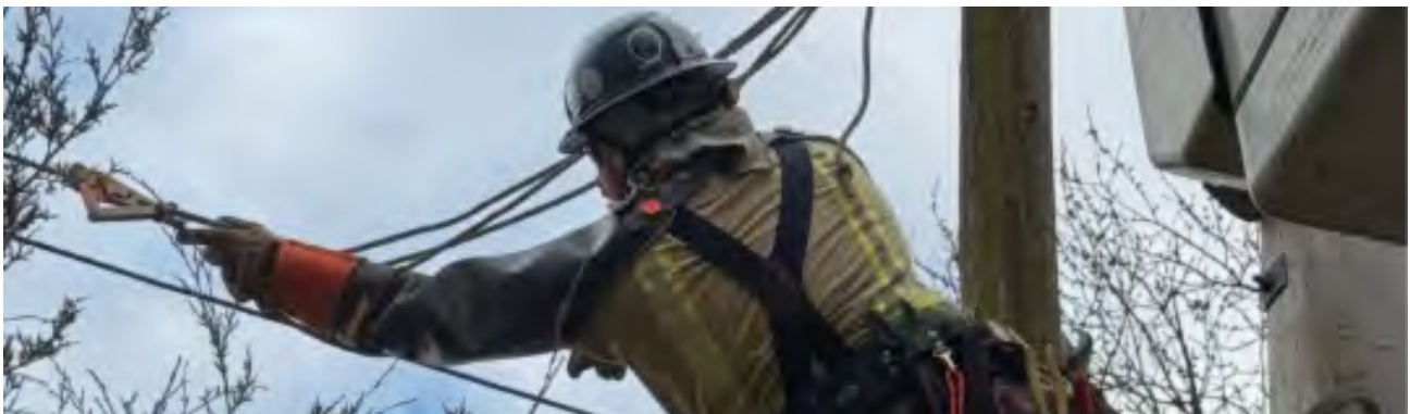
Various Electric Department project around the village.
